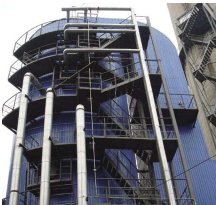
Sulphur dioxide absorber, Jinling Project in Shandong Province
