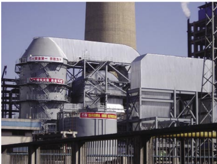
Sulphur dioxide absorber, Zhanjiang Project in Guangdong Province
