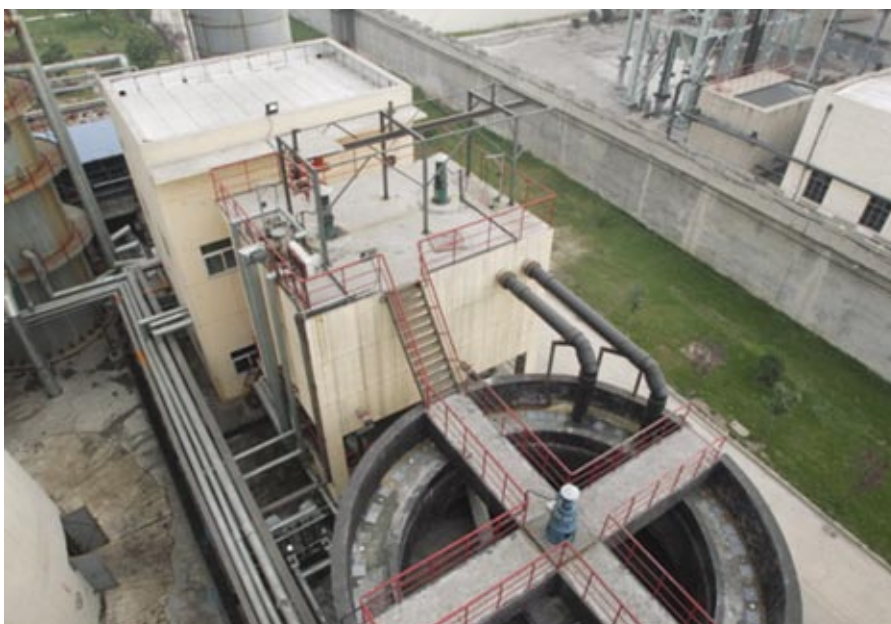
Calcium sulphite sedimentation pool, Liyang Project in Shandong Province
