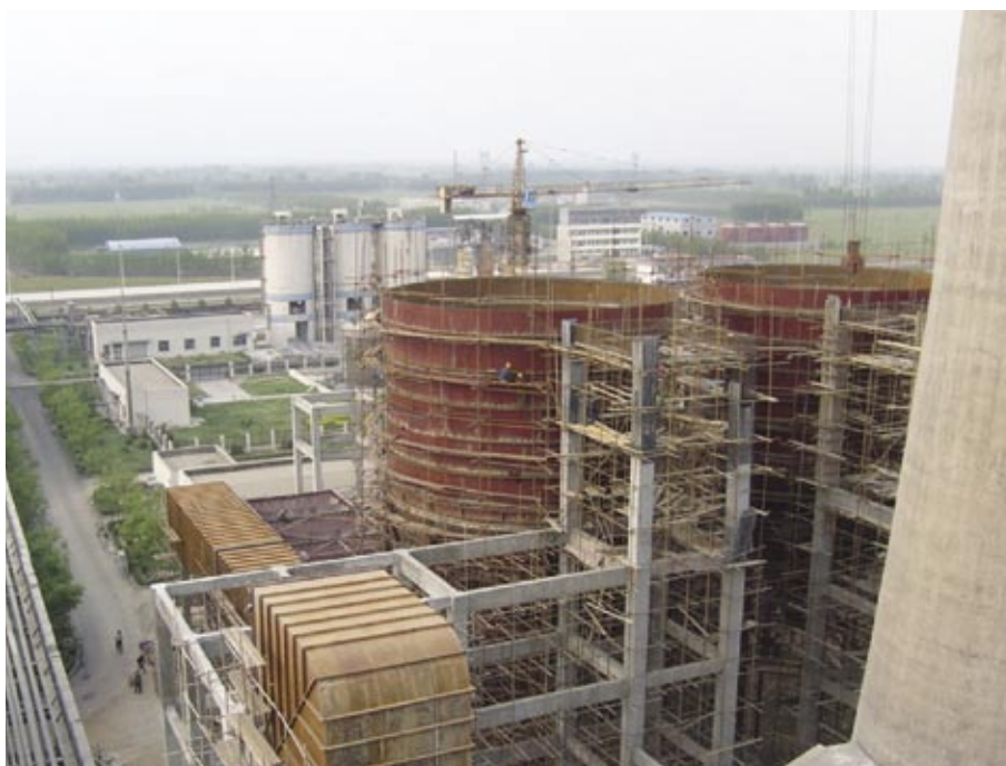
Spray Drying Absorber (SDA), Jinguan Project in Henan Province
