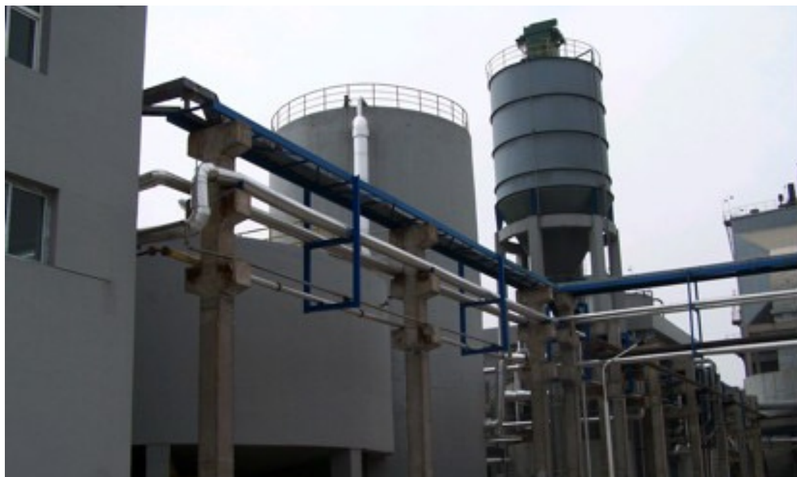
The project panorama of CNPC Lanzhou Petrol Chemicals 1×145T/H 2×220T FGD in Gansu Province Technology: TFGD
